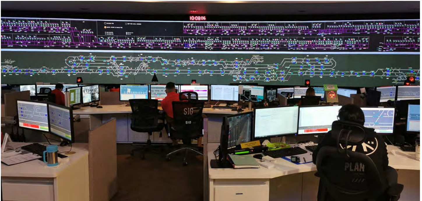
Singapore LTA's ATS is a complex, service critical system.
